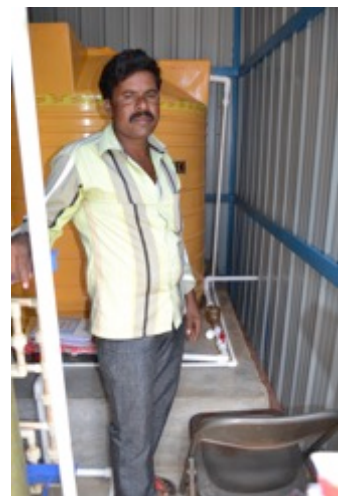
Photo 3 Rajappa the waterman showing off the Kothekote water plant
